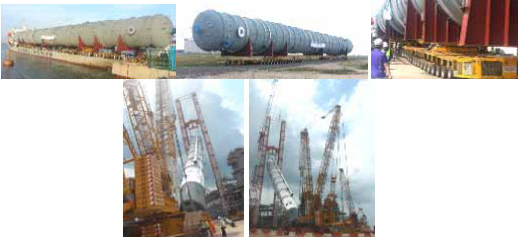
FIGURE 9: TRANSPORTING AND INSTALLING ONE OF ASIA'S TALLEST AND LARGEST XYLENE SPLITTER COLUMNS AT JAC
